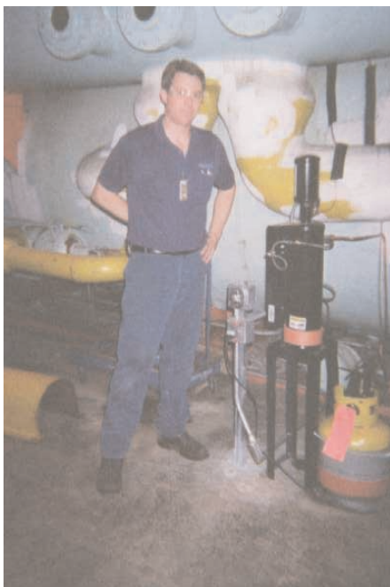
OAM-Purgers installed by Greg Beyer, Service Technician and David Holmquist, Technical Manager Central Chillers, from Owens Service Company, on a 5,500 ton chiller and on a 3,500 ton chiller at 3M facility Minnesota
